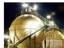
Tankanlagen Tank systems
